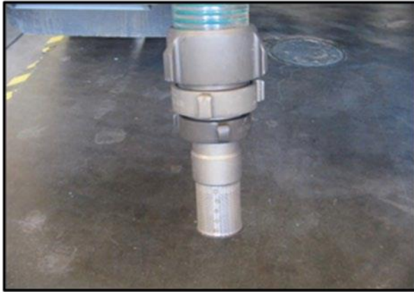
Figure 11: Foot valve attached to suction line with various adapters as needed to adjust for foot valve size
