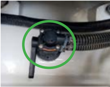
Ballast Intake Valve
