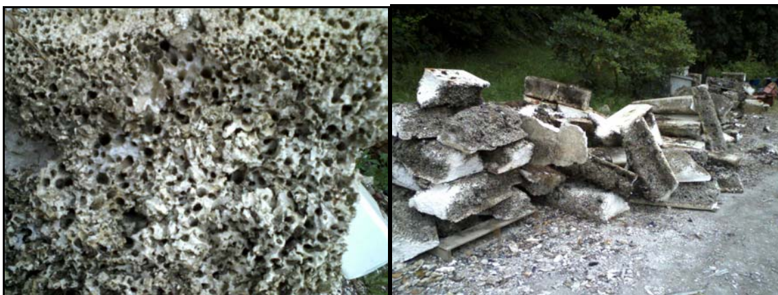
Figures 3A-B: Extensive burrowing by populations of S. quoianum (left) virtually destroyed the Styrofoam billets (right) in the floating docks used by Oregon Oyster (Newport, OR).
